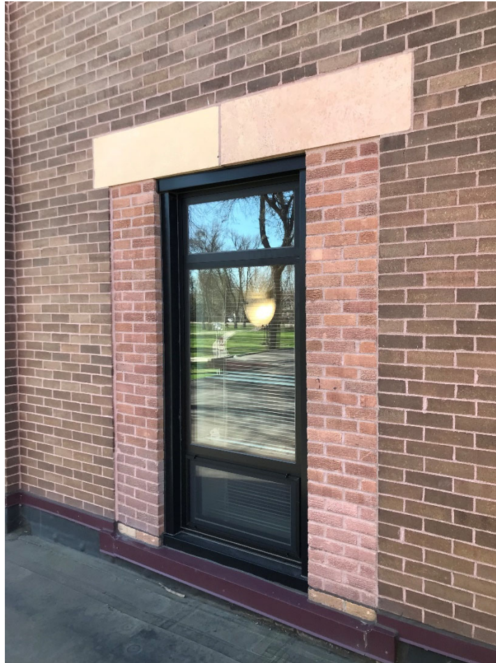
Graham Hall Exterior Photo at Level 2 – existing opening at new V200 HM door location
